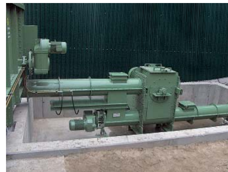
Shredder integrated in the conveyor system
