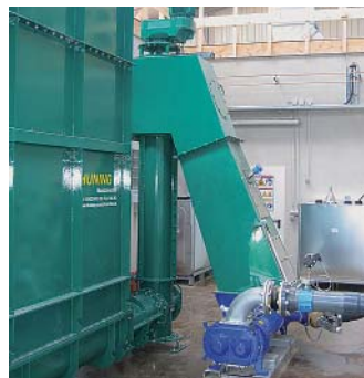
Transfer from the solid matter dosing system into pump systems
