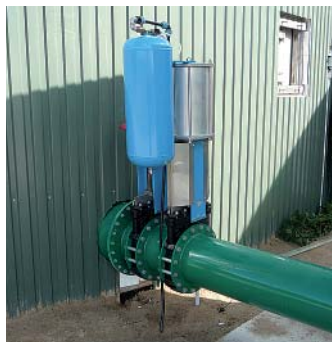
Direct feeding from the solid matter dosing system into the fermentation plant
